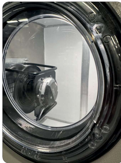
AHU fan viewed through porthole.
