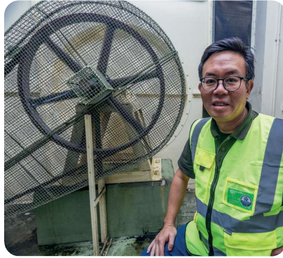
DRLC staff member Gary next to air handling unit.
